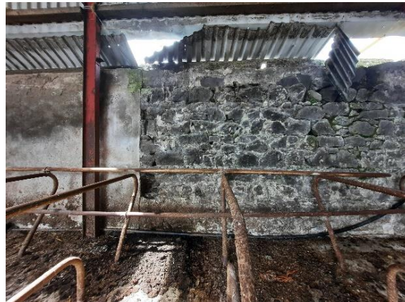
Plate 4-10 Stone wall with crumbling cement and gaps
