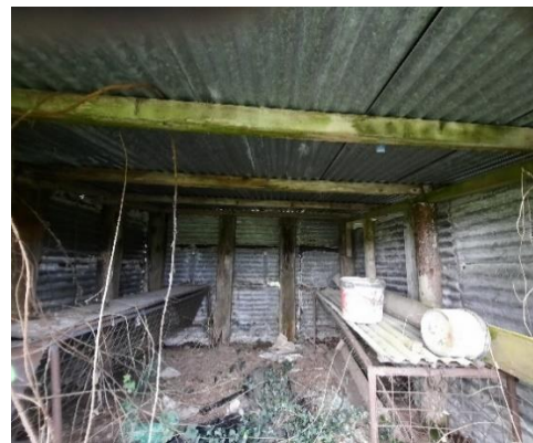
Plate 4-6 Southern section showing old hay feeders and rubbish with ivy and briars growing through the sheets
