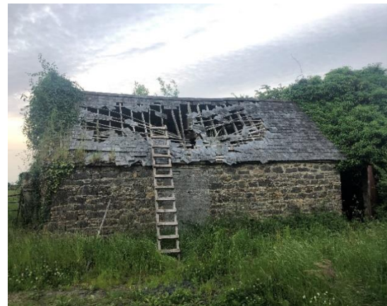
Plate 4-2 Stone shed with roof damage and ivy cover
